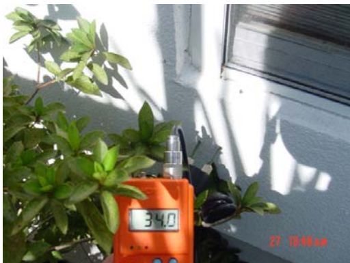
Detail Photo #5 -- No sealants at window lower left. High moisture reading at this window. Seal perimeters/construction.
