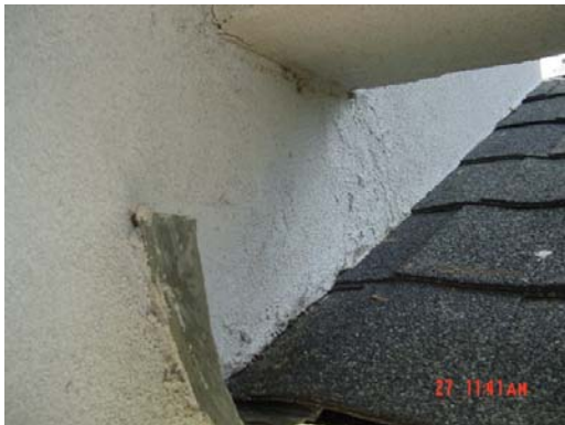
Detail Photo #9 -- Kickout flashing is present. This was installed after original EIFS installation. Noticeable patch. Seal.
