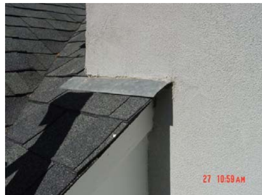
Detail Photo #6 -- EIFS is flush on roofing/flashing. Modify to prevent moisture intrusion.
