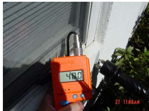
Detail Photo #12 -- No sealants at window lower right. High moisture reading. Seal perimeters/construction.
