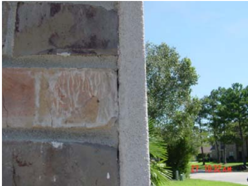
Detail Photo #1 -- Brick Terminations. No sealants present. Seal all brick/EIFS terminations to prevent moisture
