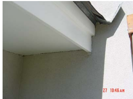
Detail Photo #4 -- No sealants at soffit/fascia. Seal all soffit/fascia areas to prevent moisture intrusion.
