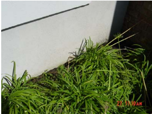
Detail Photo #7 -- Lower Edge. Landscaping is too close to foundation grade. Assess and modify.
