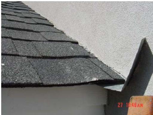
Detail Photo #3 -- EIFS is flush on roofing. Consult a qualified waterproofing contractor to modify.
